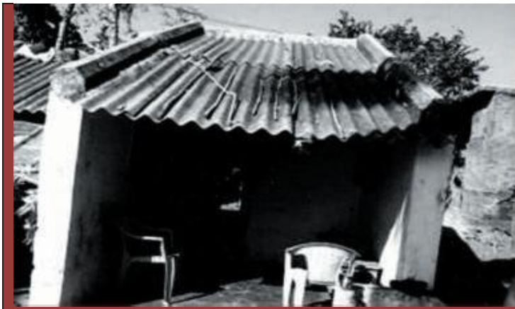
Exhibit 4.6 Dilapidated Anganwadi Centre building in Project Parvathipuram, Vizianagarma district, Andhra Pradesh
